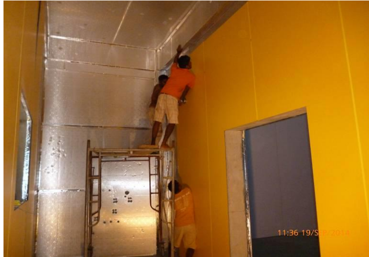
Front Air corridor of the Laboratory (air corridor)
