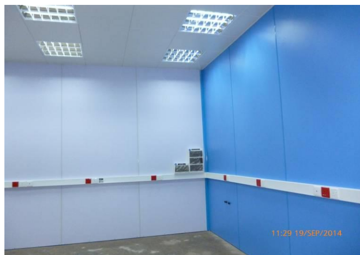
Thermal protection inside the walls of the laboratory and Electricity supply unit
